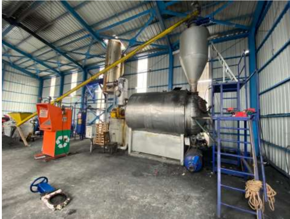
Figure 2. Pyrolysis Facility of Karabuk Municipality
